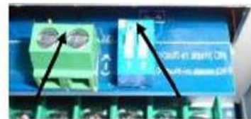
Terminal strip J22 Toggle switches
